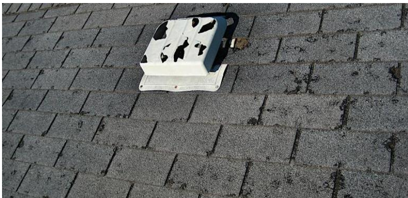
Roof needs to be replaced
