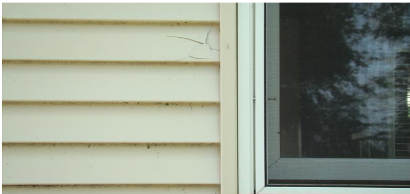
Cracked exterior siding
