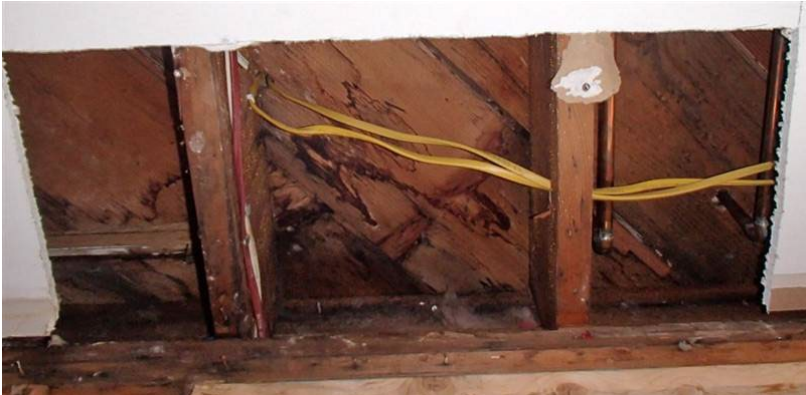
Water damage to main floor
