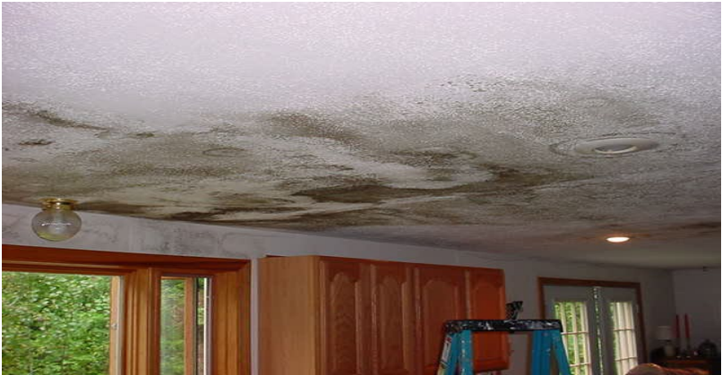
Water damage to main floor ceiling
