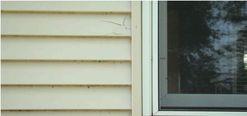
Cracked exterior siding
