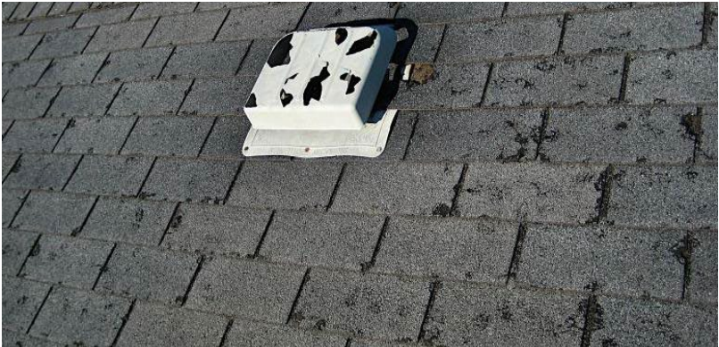
Roof needs to be replaced
