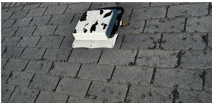
Roof needs to be replaced
