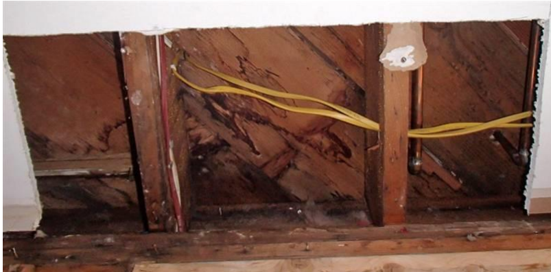
Water damage to main floor
