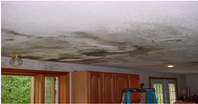
Water damage to main floor ceiling
