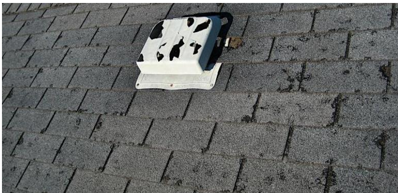
Roof needs to be replaced
