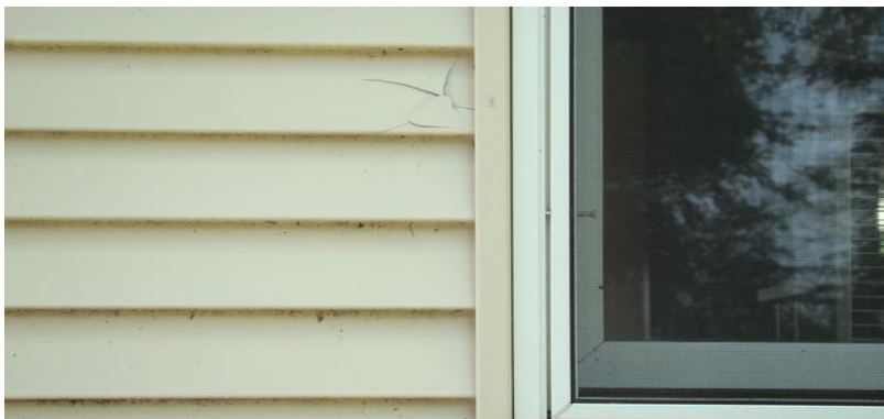
Cracked exterior siding
