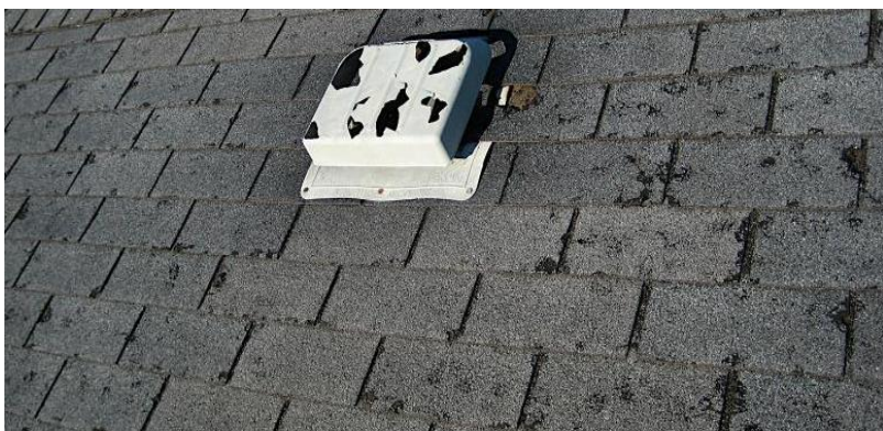
Roof needs to be replaced
