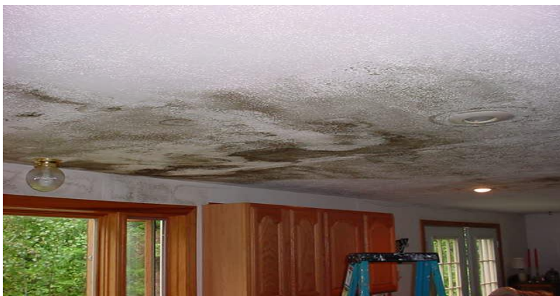
Water damage to main floor ceiling
