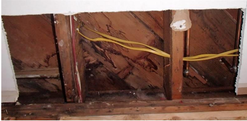
Water damage to main floor
